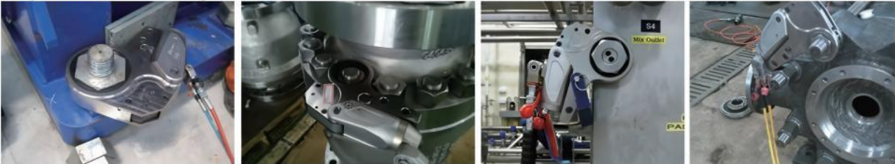
客戶現場工況實例: Example of customer's on-site working conditions:
