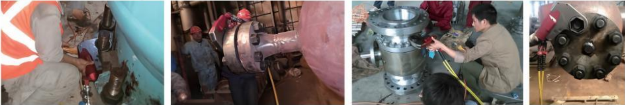
客戶現場工況實例: Example of customer's on-site working conditions:
